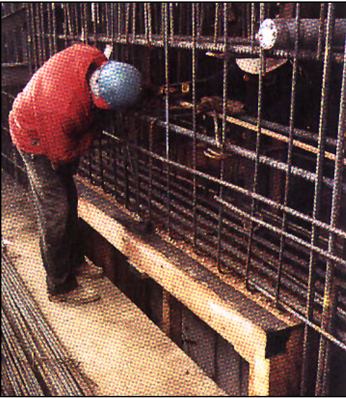
Figure 3. Greater spacings between yokes give contractors more room to place blockouts for openings and connections in structures. Greater clearances also give workers more time to place horizontal rebar before the next layer of concrete is placed in the slipform.
